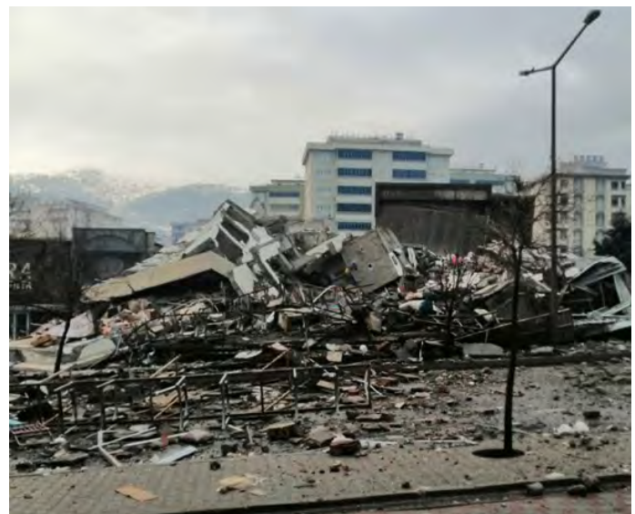
Figure 2. View of a collapsed building in the city center of Kahramanmaraş (photo by Dr. Yavuz Orak).
